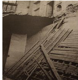
Fig (4) The collapse of the timber in house of Ali katkuda after the earthquake 1992 (JERE L1995)
